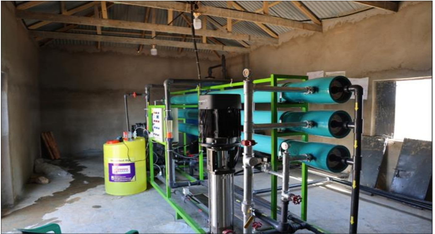
Fig 1 Installed Desalination Plant in El-dahir Village, Somalia
